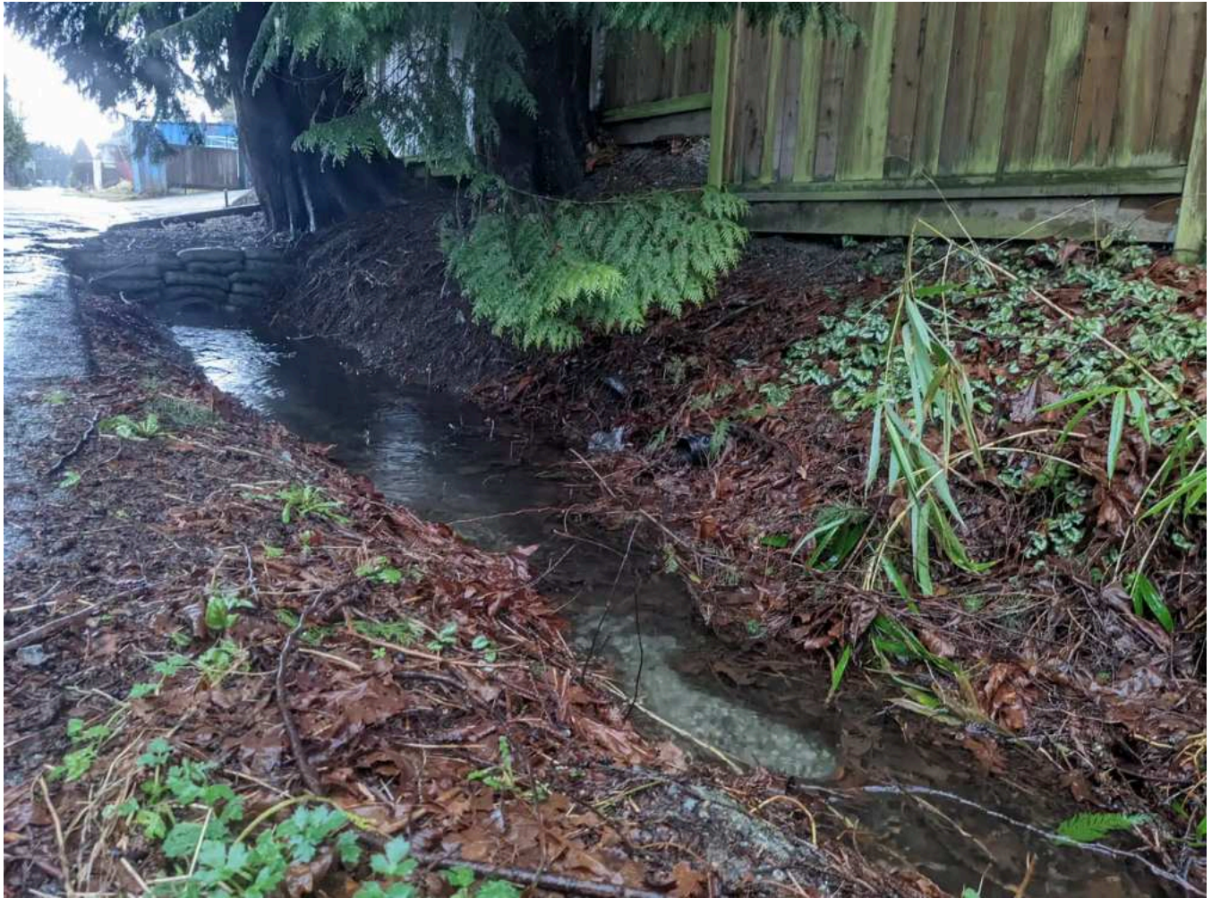
Figure 6.1.7: Image of the open culvert at East end of Edgar Avenue during rainfall.
